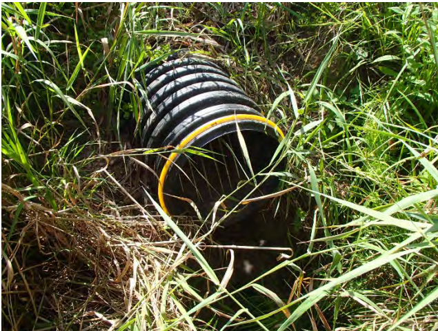
CV004TMM Bearing: OUTLET Date: 09/11/2019
