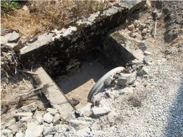
CV002TMM Bearing: INLET Date: 09/11/2019
