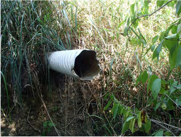
CV006TMM Bearing: OUTLET Date: 09/11/2019
