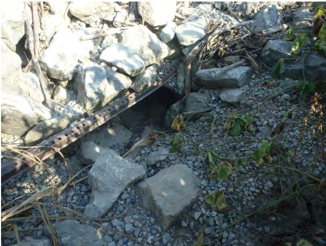
CV008TMM Bearing: OUTLET Date: 09/11/2019
