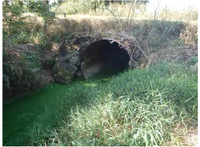
CV001TMM Bearing: OUTLET Date: 09/11/2019
